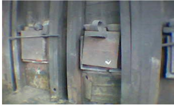
Figure 1.11 Door in a Furnace
