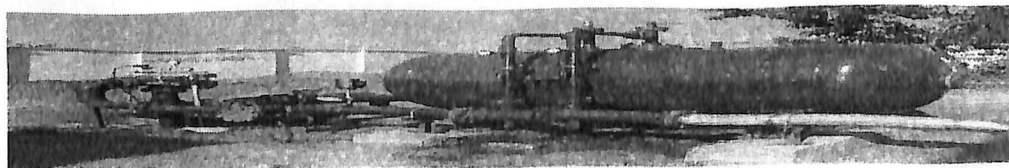
Fig 09:- Foam Flooding System
