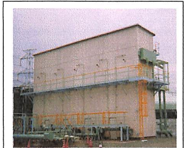
Figure 6.15: Forced air Circulation LNG Vaporiser
