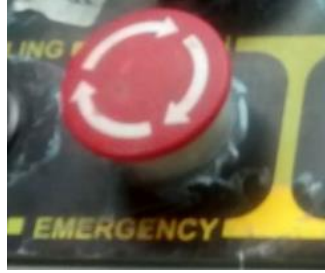
Figure 22: Emergency Push Button
