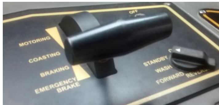
Figure 23: Emergency Brake in Master Controller
