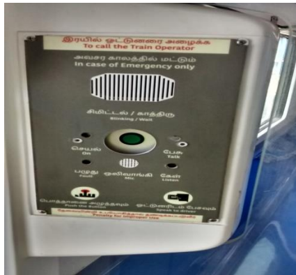
Figure 13: Passenger Emergency Intercom
