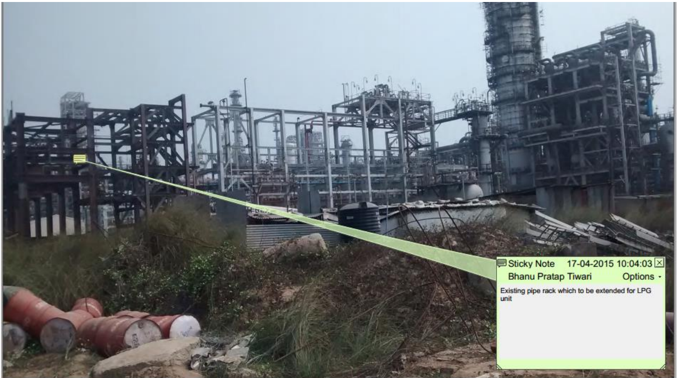
Figure 5.7: Existing Pipe Rack to be extended for LPG Unit
