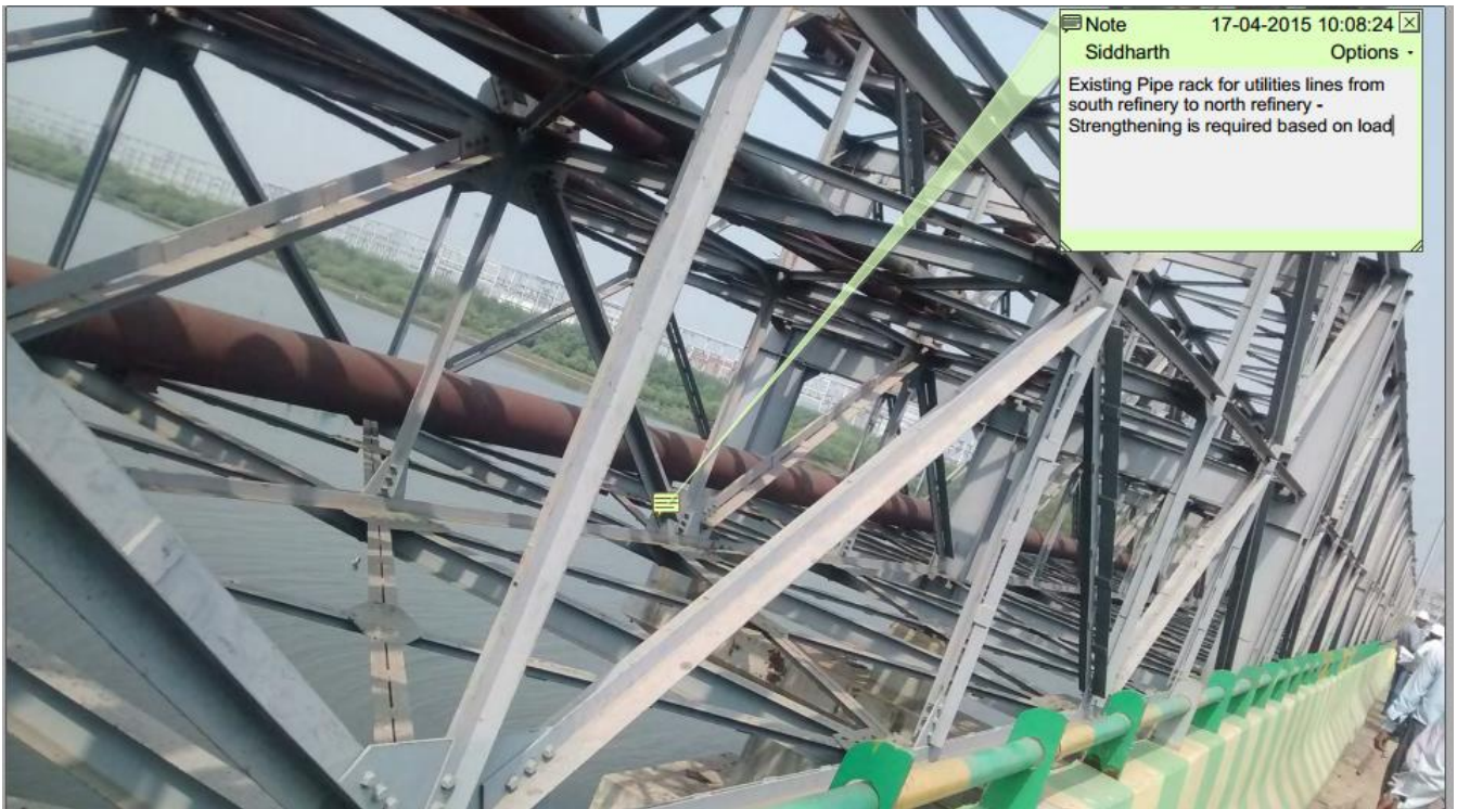
Figure 5.8: Existing Pipe Rack for Utilities
