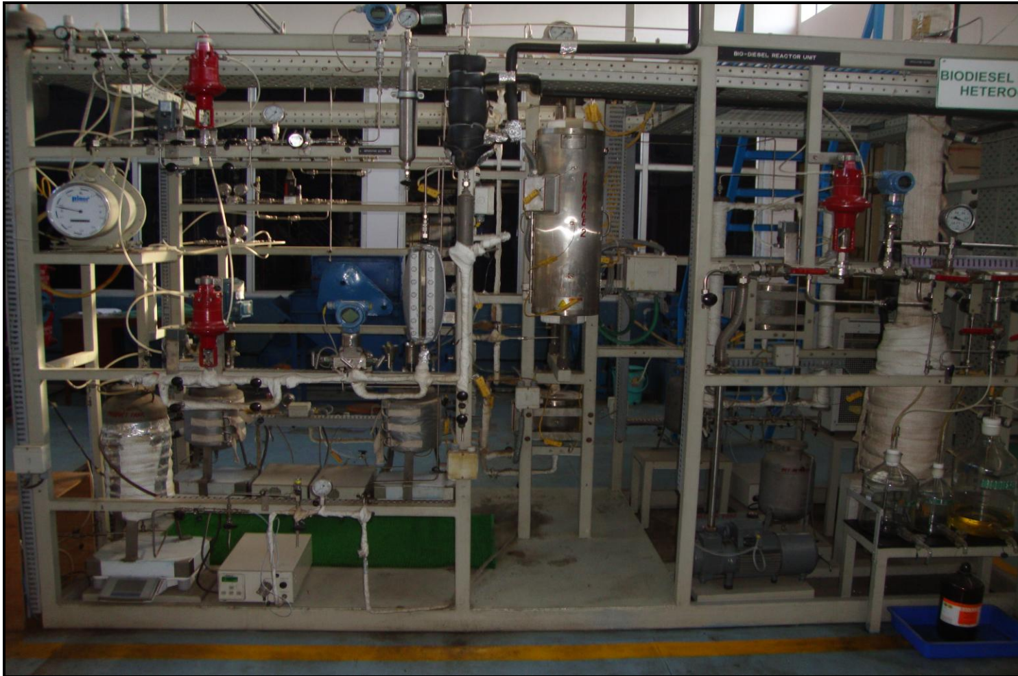
Fig. 6.2: Front view of biodiesel pilot plant
