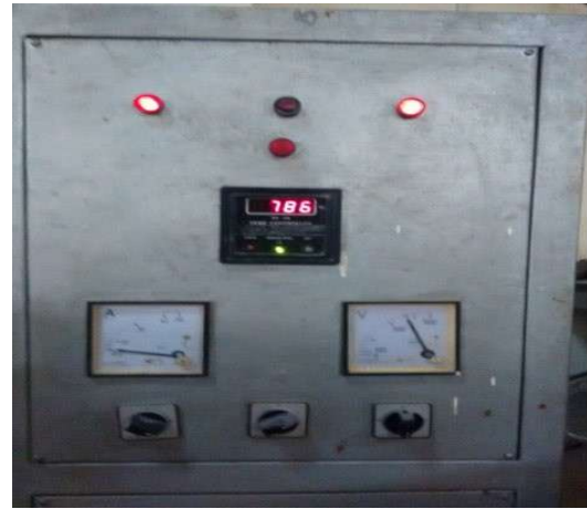
b) Furnace controller
