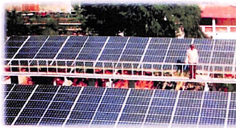
Figure 2.4: SPV Power Plant
