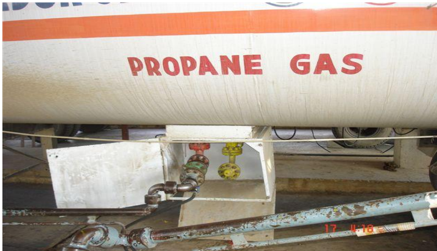
Figure 5– Tanker with Liquid and Vapor connection
