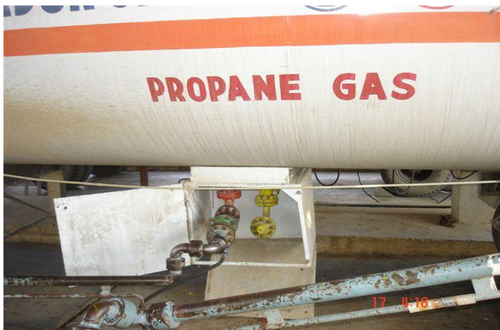
Figure 13 - LPG / Propane tanker with liquid line connection
