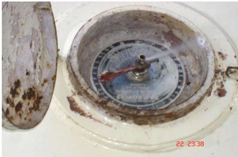
Figure 2 – Releasing LPG /Propane from Rotogauge
