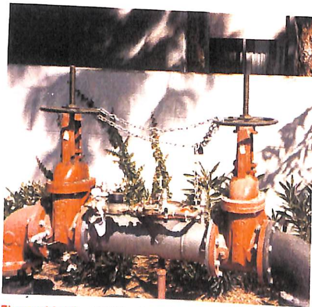
Figure 12-13 OS&Y valves chained in the opened position.
