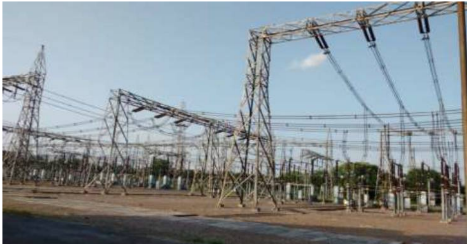
Fig 2.2 Air Insulated Substation and Switchyard with Gravel Surface
