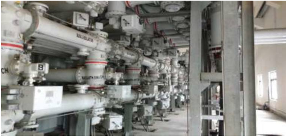
Fig 2.1 High Voltage Gas Insulated Substation
