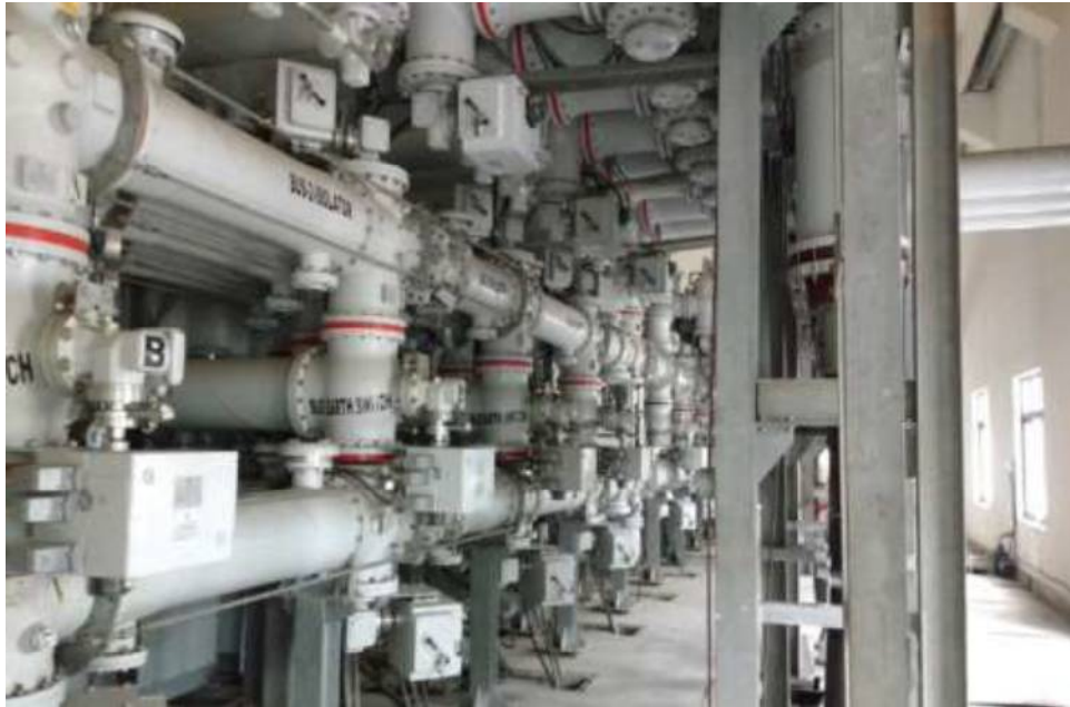
Fig 2.16 Actual View of GIS Substation
