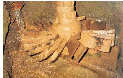
(Fig 3.6:Damaged Penstock Nozzle at a Watermill at Bhatwari dated 20.06.2008 )
