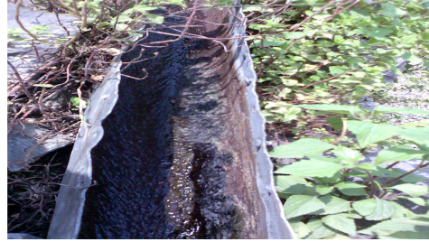
(Fig3.8:Breached Channel at a site in Bhimtal dated 28.06.2008 )
