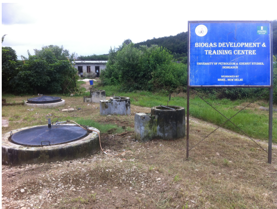
Figure 3.1: Cow dung based Anaerobic digester plant in UPES, Dehradun
