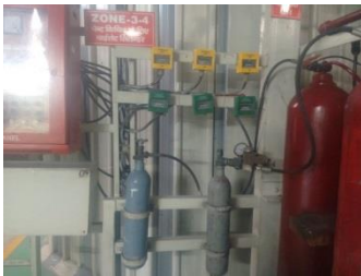
Fig 4.3: Pilot cylinders for paint kitchen
