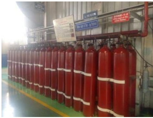
Fig 4.1: CO 2 Flooding System
