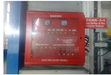
Fig 4.2: CO 2 control panel
