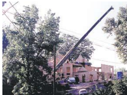
Fig 3.5 Operating a crane near overhead wires is very hazardous
