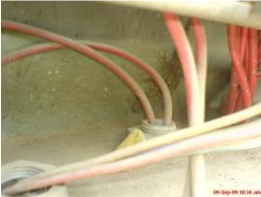
Fig 4.6 No dustproof and water proof condition
