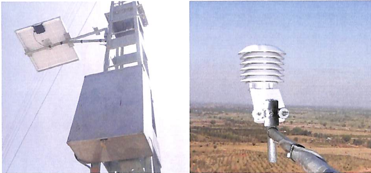
Figure 20: Wind Mast & Temperature Sensors.
