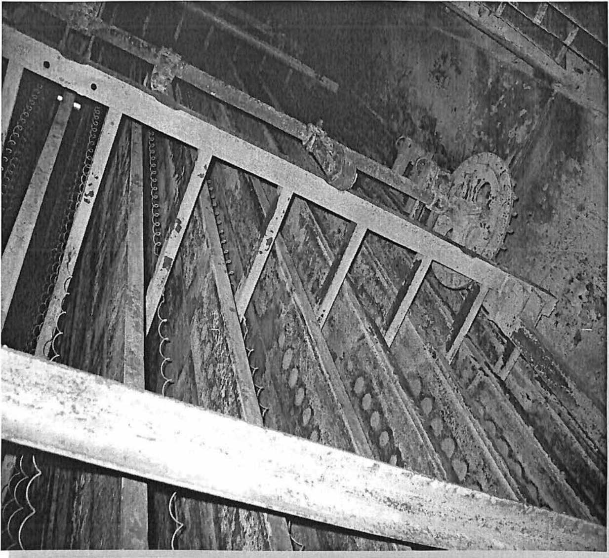
Inside view of E.S.P
